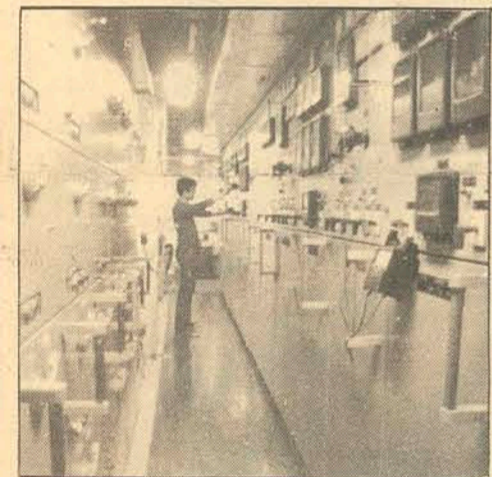
Painel de controle
